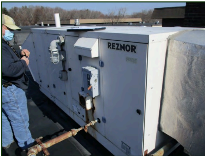
Current Rooftop Units
