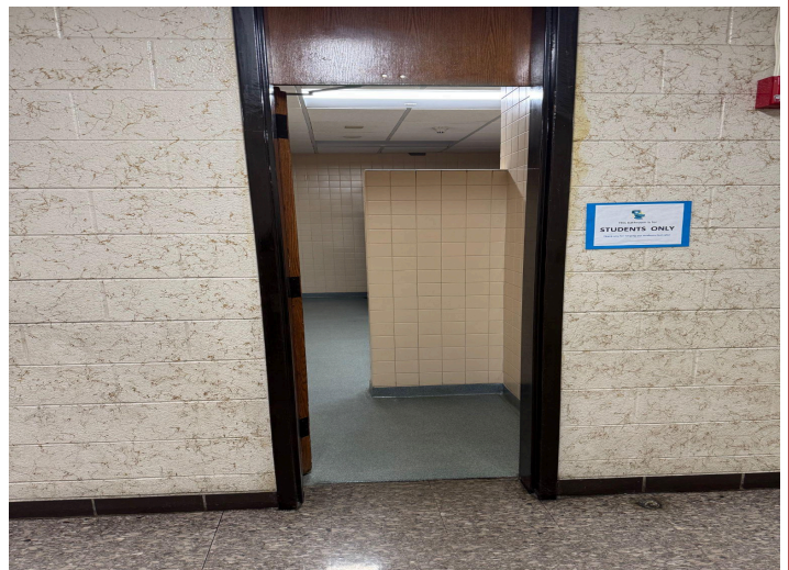
Doorway is 10" under code
