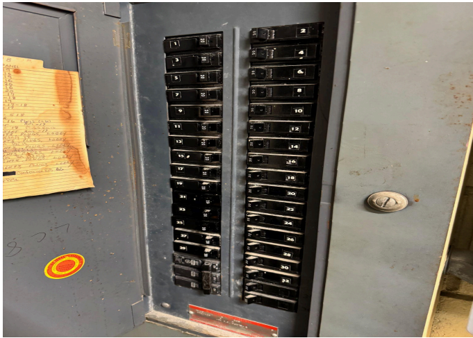
Outdated Electrical System
